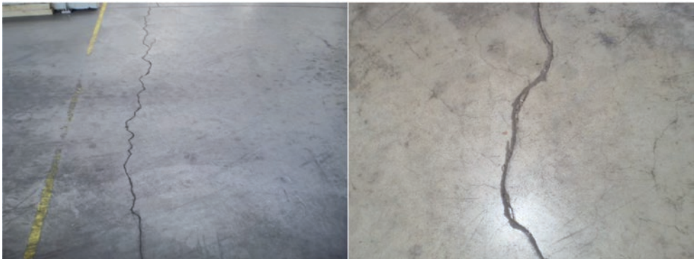
Figure 5 Cracks near the entrance (V1 and V2)
