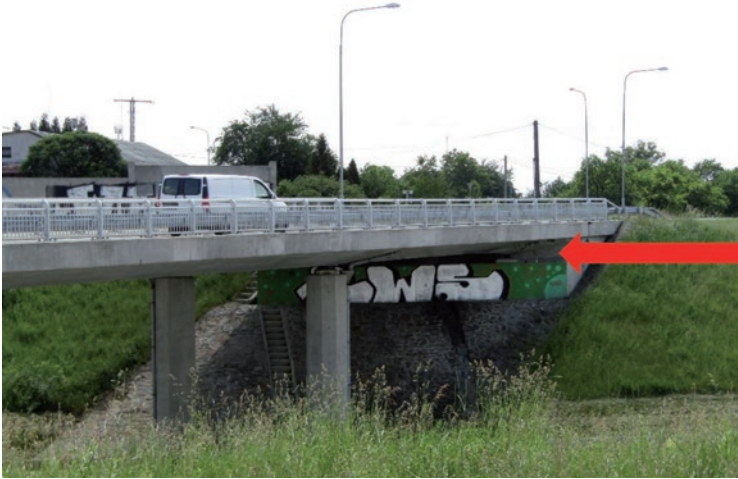
Figure 10: The concrete bridge structure under the street Ostravská (located above the bridge D1)
