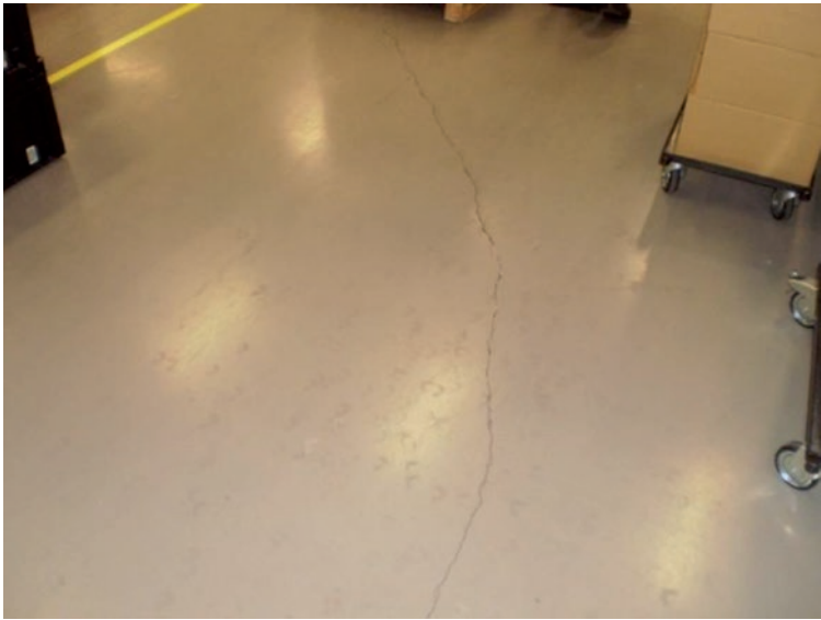
Figure. 10 Cracks on the floor
