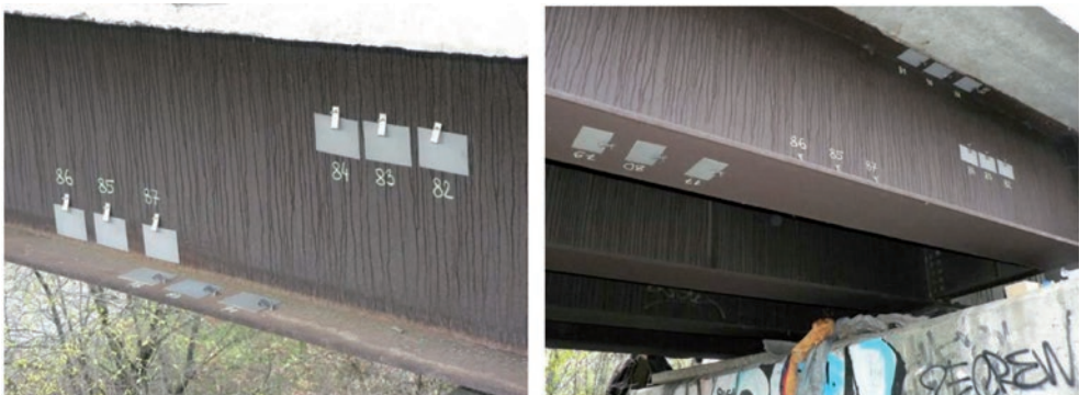
Figure 3: The installation of corrosion specimens on the railway bridge in Prague - Motol
