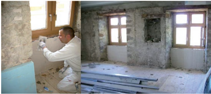
II.1. The application of aerosol insulation in the place of external wall tinning (EnergieCluster. HLWD Course 2011 Innendämmung mit Aerogel. Training materials 2011).
