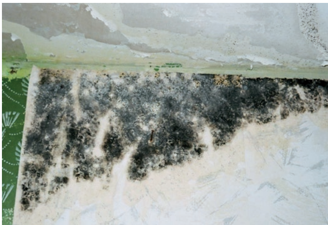
II. 3. Moulds on a wall of a room under the ceiling - after "flooding" (the author).
