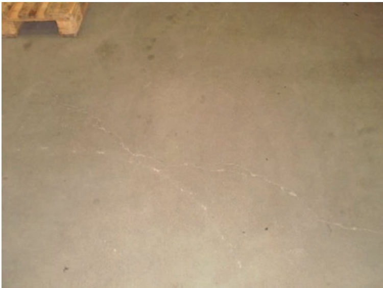
Figure. 11 Cracks on the floor
