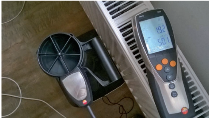
Figure. 2 Controlling of flow volume on outlet (Testo 435-2, anemometer and Testovent 417)
