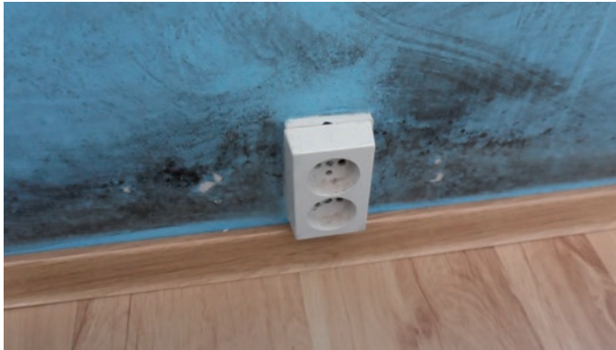
II. 2. Moulds around an electrical socket and skirting board on the ground floor (the author).
